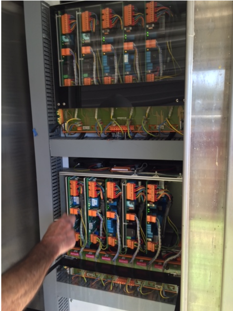
FIGURE 2.4 CONTROL CENTER – BALLAST CABINET
